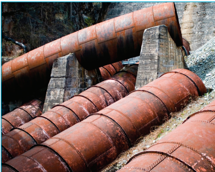
Water pressure: utilities are turning to smart technology to detect leaks and to learn about how much is consumed and by whom.
