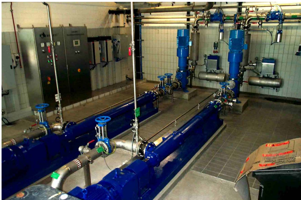
Siemens Crown Disintegrator Wiesbaden WWTP - 60m 3 /hr
