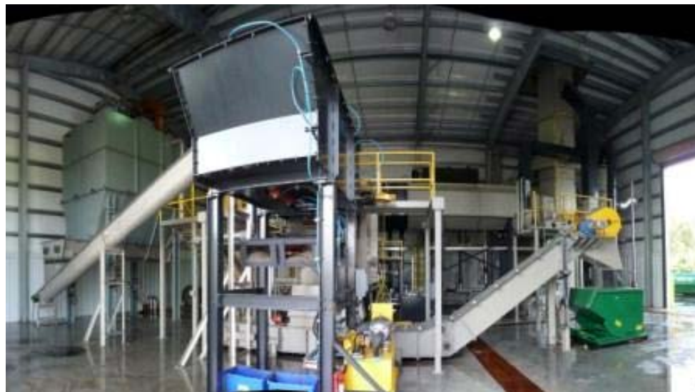
MaxWest System – Sanford, Florida
